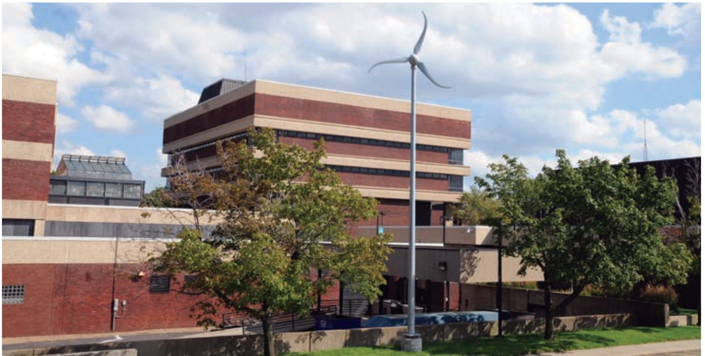
Metropolitan Campus Wind Turbine
